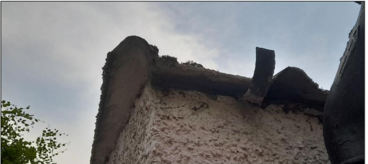
Photo 2: Gap at another corner
