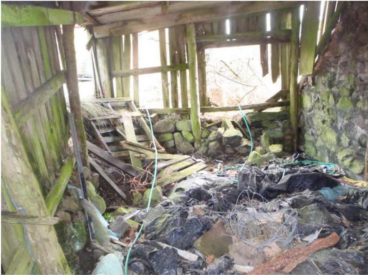
Photograph 6: showing a view of the lean-to structure located north of the main building
