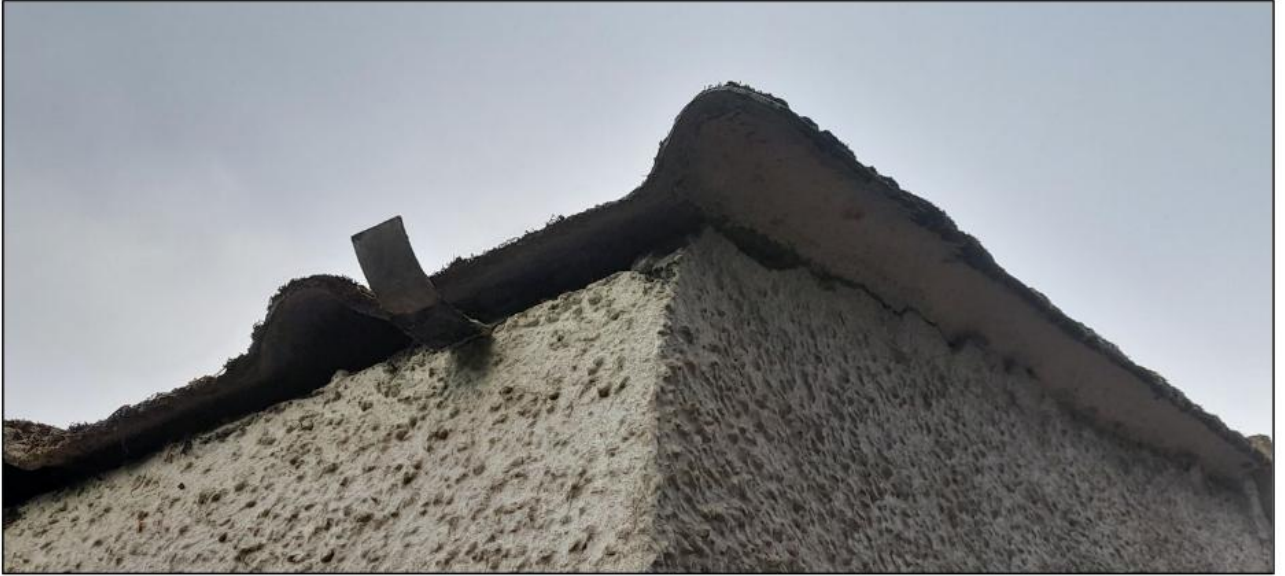
Photo 1: Gap at one of the corners of the garage
