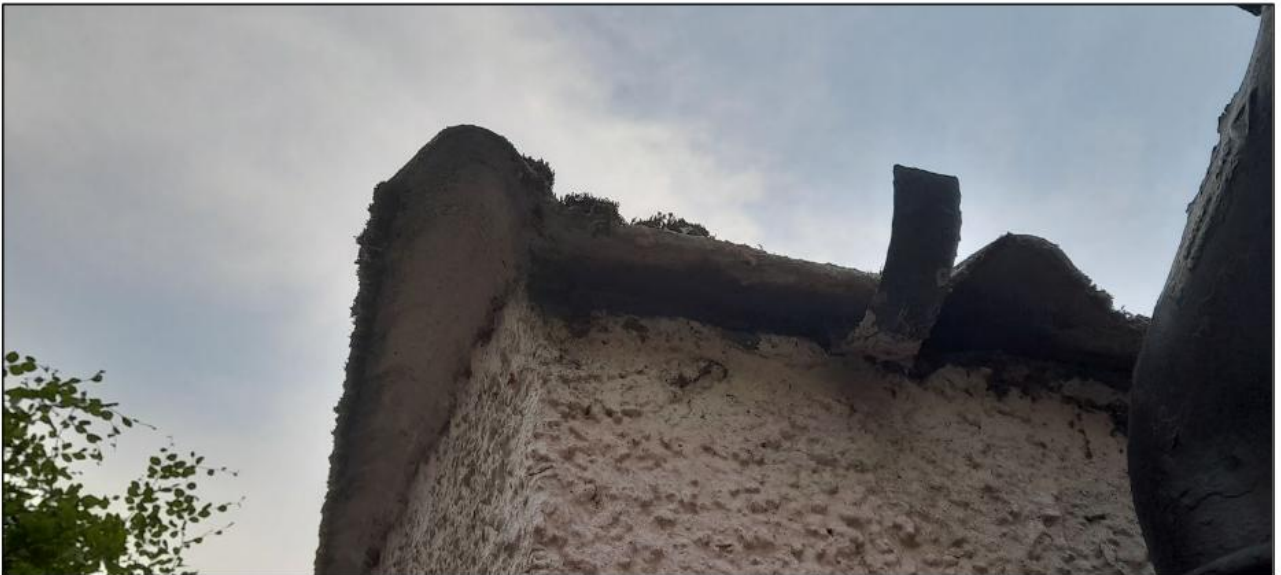
Photo 2: Gap at another corner
