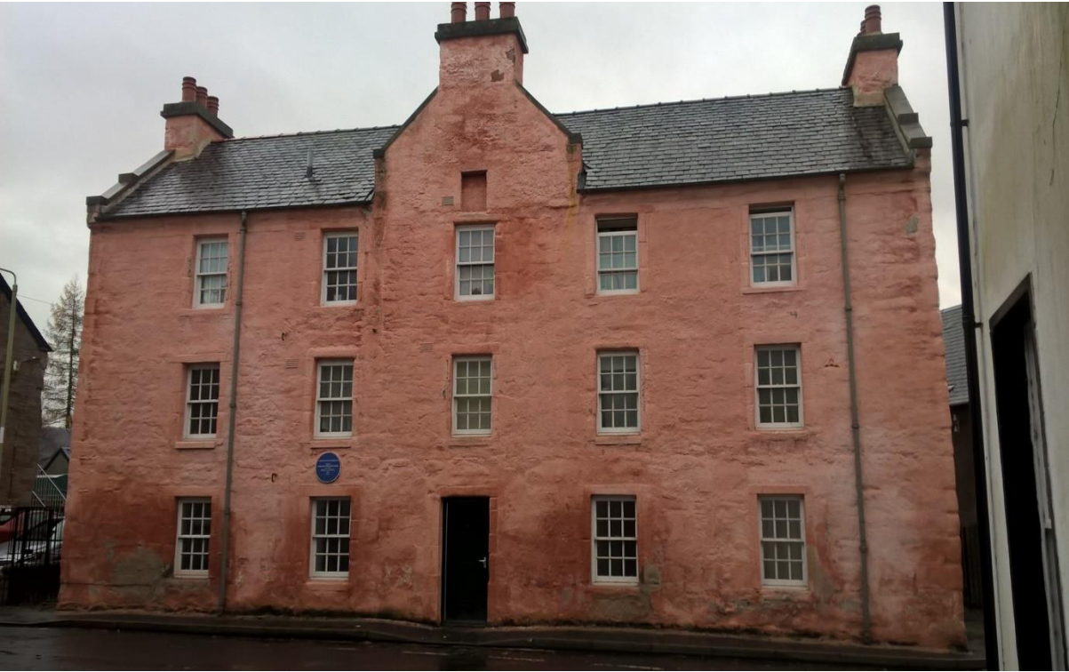
Pictures of Cumberland Barracks before the improvement works:
