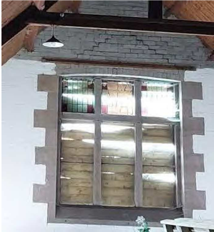
Figure 5: Example of Inverted V Shaped Cracks over Windows
