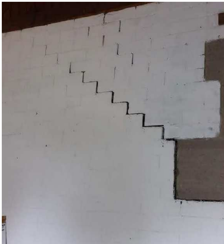
Figure 6: Example of Cracking from Excessive Settlement in External Walls
