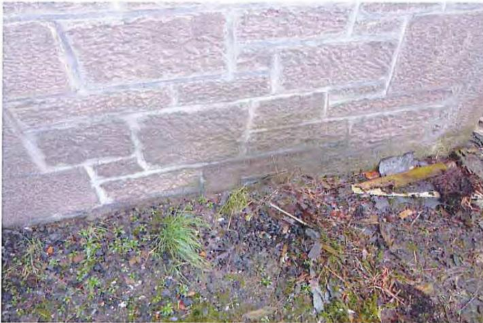
17 Hall: blocked underfloor ventilation.
