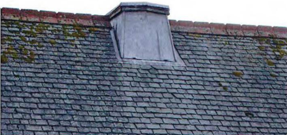
8 Capped ridge ventilator – no ventilation to Hall .
