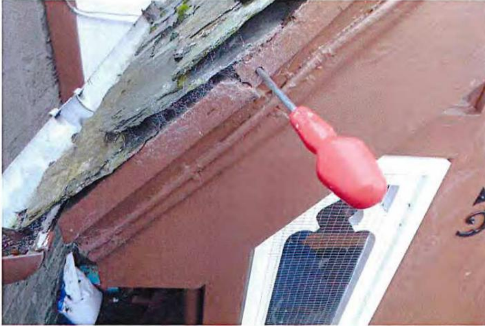
11 Rot in gable bargeboards/bending.
