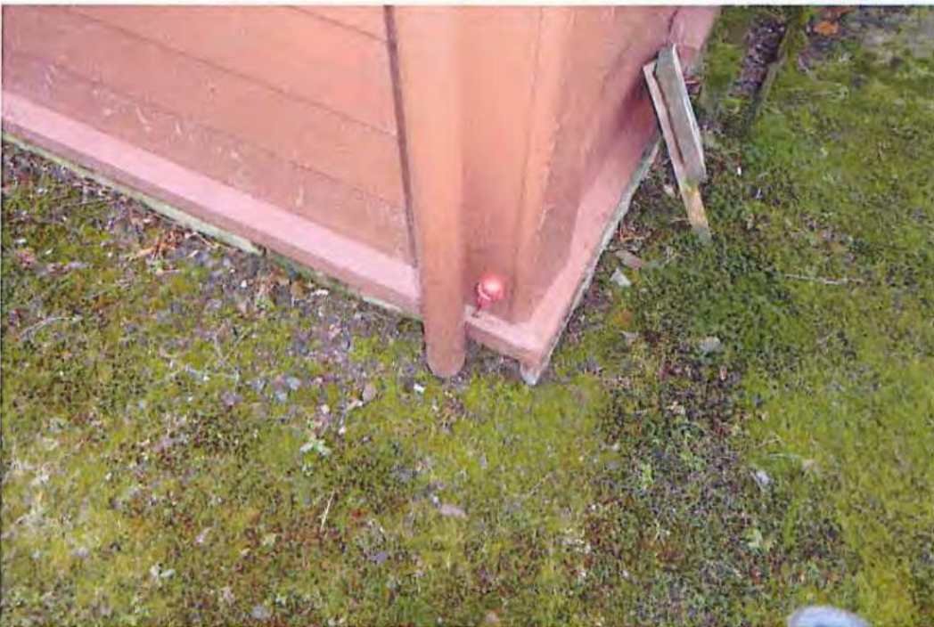
2 Wet rot in timber 'cill' at most corners.
