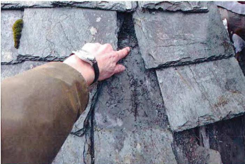
12 Slates eroding at nail holes; slate slipping.
