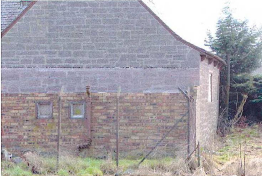
31 Hall: East gable: partially demolished outhouses. North wall bulge/cracking
