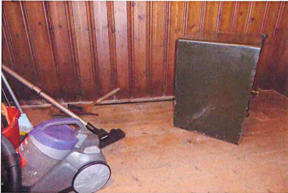
21 Sag in vestry floor; heavy safe/floor loading.
