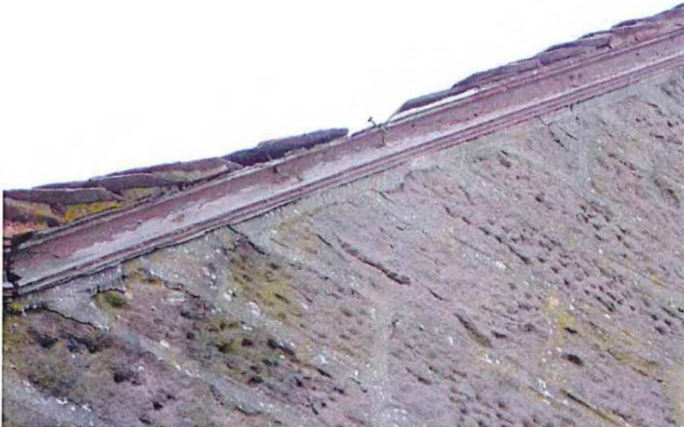
25 Hall gable – missing slate, poor verge pointing, rot in gable timbers.
