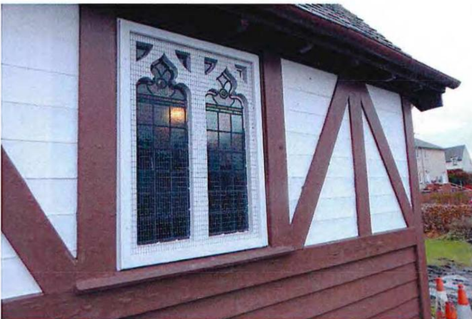
4 Blistering and wear to paintwork.
