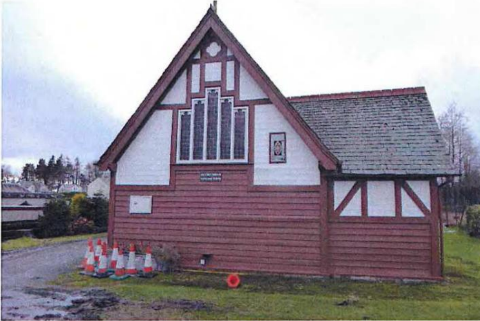
5 East elevation; split/warped weatherboard.
