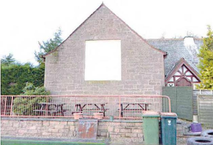
24 Hall; south elevation. Water run-off.
