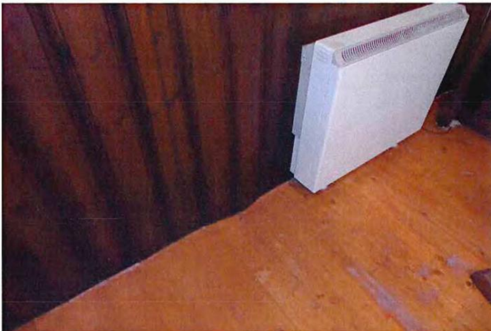
20 Swollen and buckled timber dado lining.
