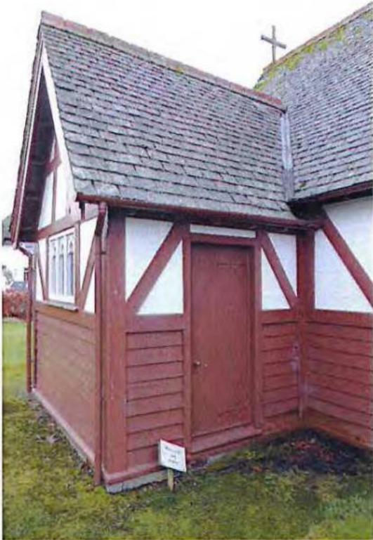
15 Vestry back door; leaks/overflow, patched lead valley at roof junctions.
