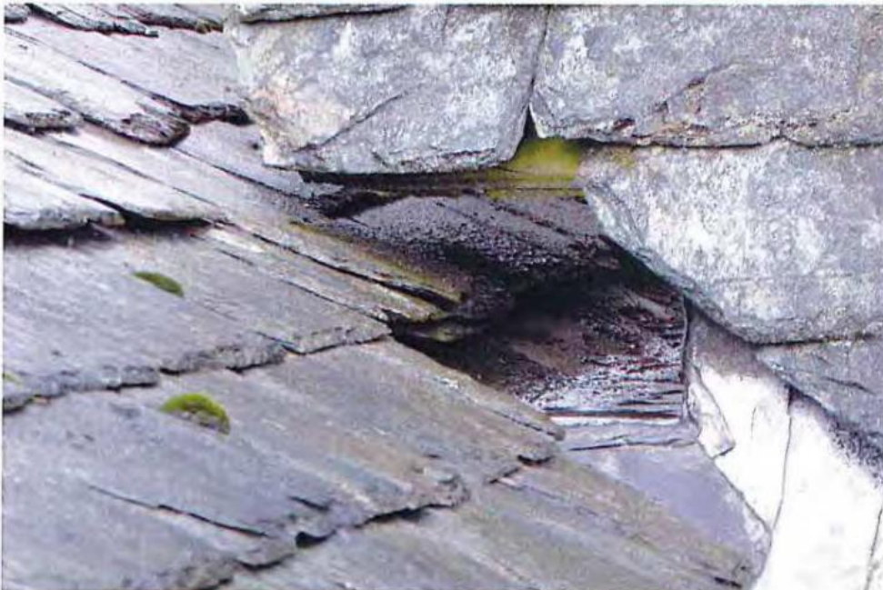
10 Leaking tapered lead gutter at Church/Hall roof junctions.
