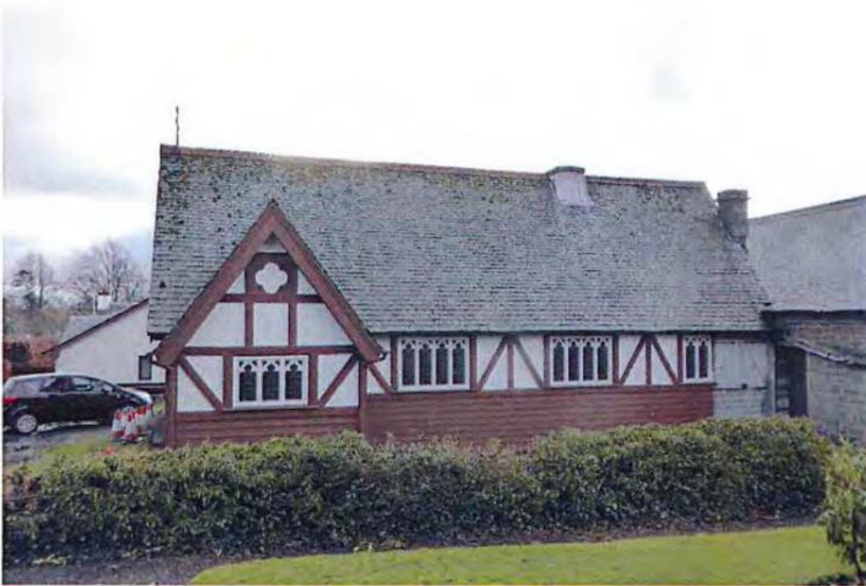
7 North elevation; moss on slate, a few slipped slates.
