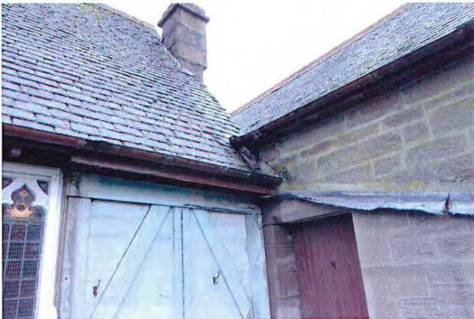
16 Water penetration; leak at roof junctions; vulnerable detail.
