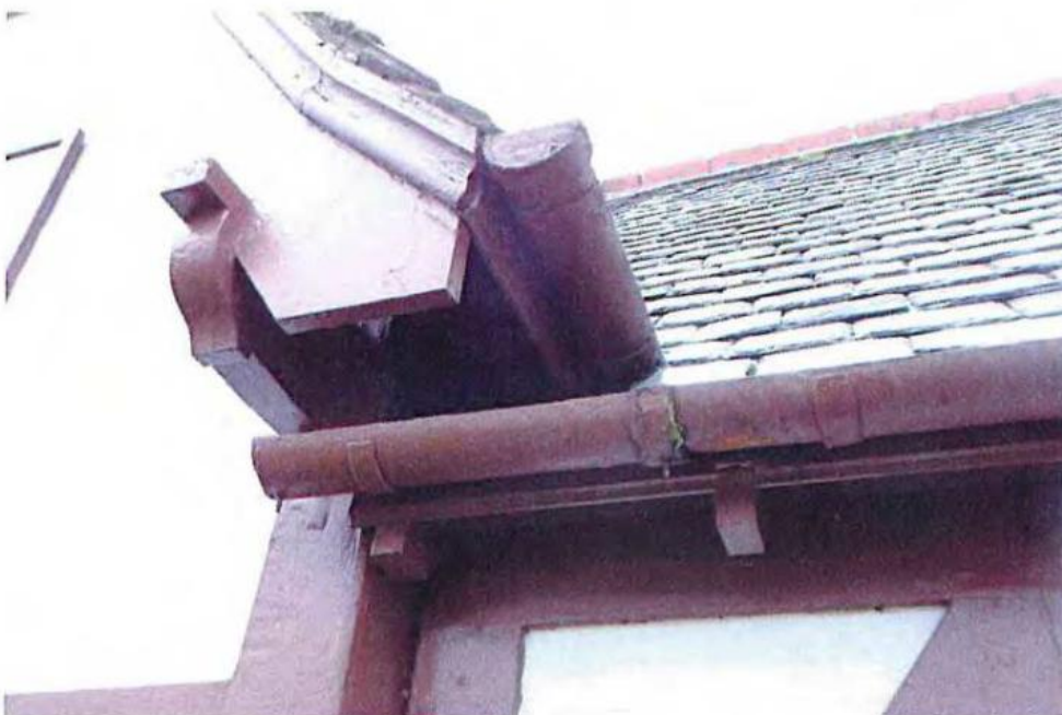
6 Leaking rainwater goods at joint.
