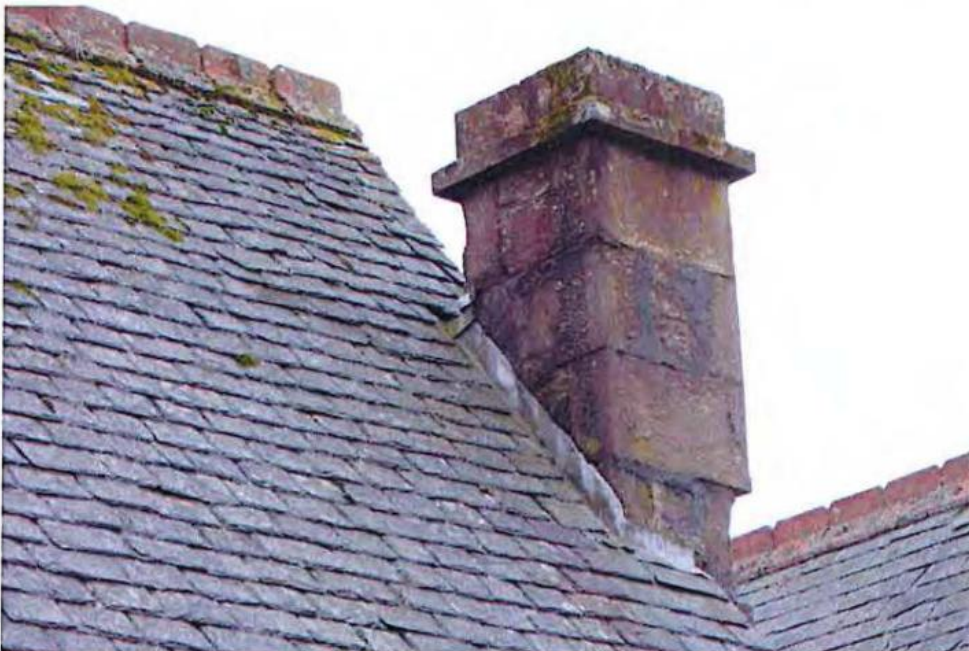
14 Deteriorated chimney and lead flashings.
