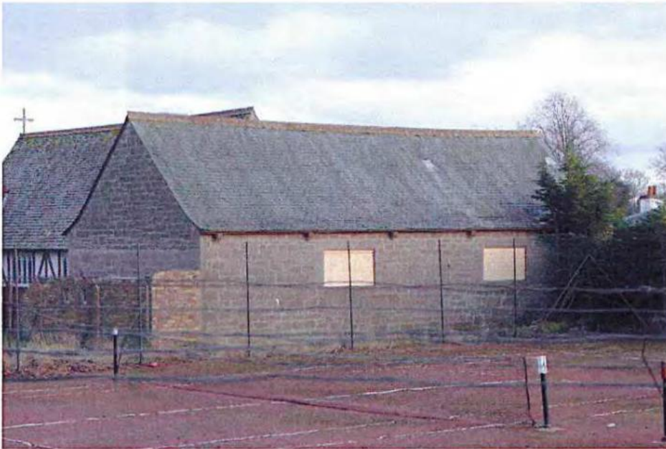
23 Hall from west elevation; boarded up windows. A few slipped slates.
