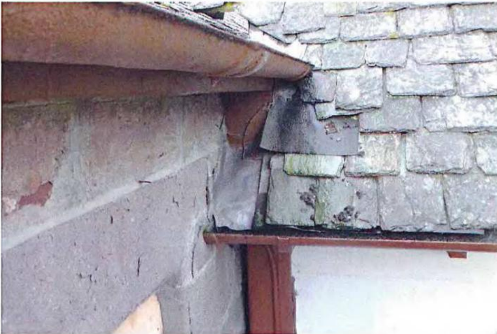
3 Gap between Church and Hall: vulnerable point rainwater discharge from Hall roof to Church roof
