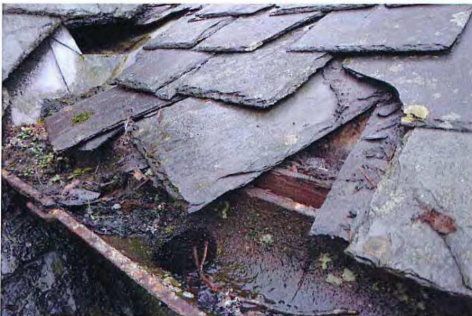
18 Hall roof; rot in base of timber sarking.
