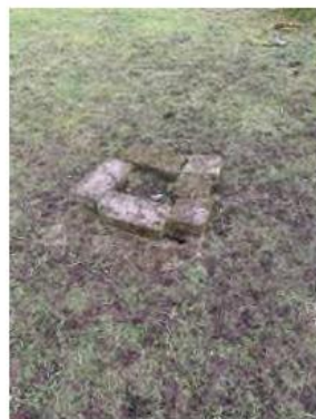
1 Mawcarse Cottage – Old Style Primary Treatment Septic Tank
