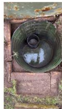
1 Mawcarse Cottage – Old Style Primary Treatment Septic Tank
