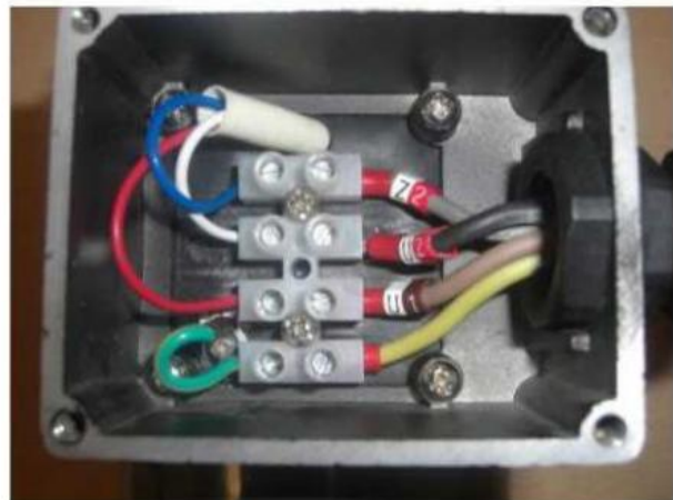
Motor Terminal Box
