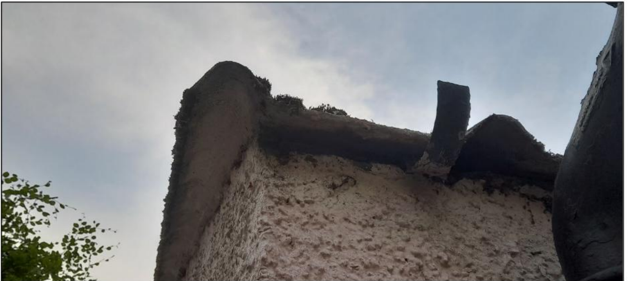
Photo 2: Gap at another corner
