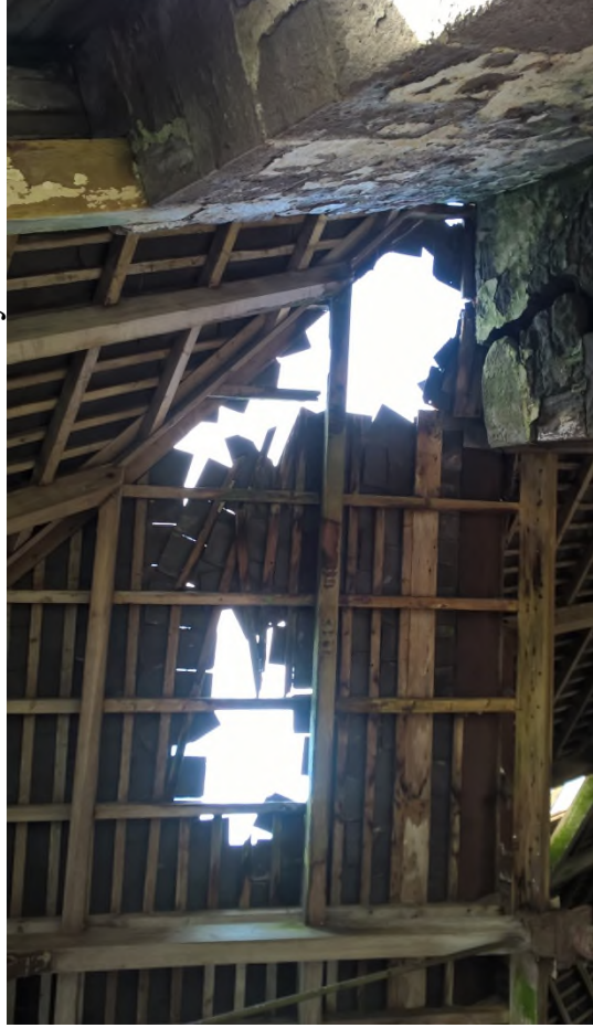
Condition of steading
