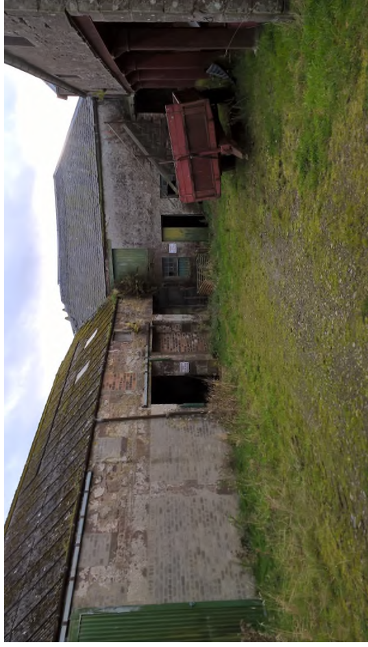
Condition of steading
